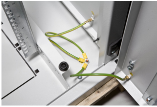
internal earthing of all cabinet parts
